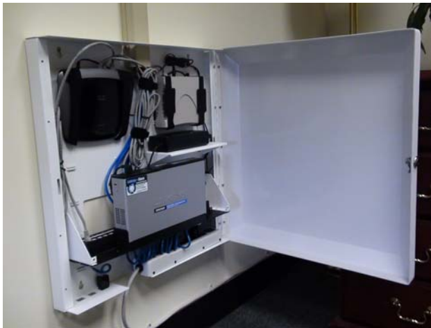
Wall mount or "reclined" router strapped to back box, rack-mounted switch and patch panel, cable modem, surge protector or strip
