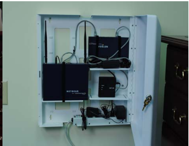
Desktop "stand-up" wireless router (note the vertical dipole antennas), switch, DSL modem, and surge protector / power strip
