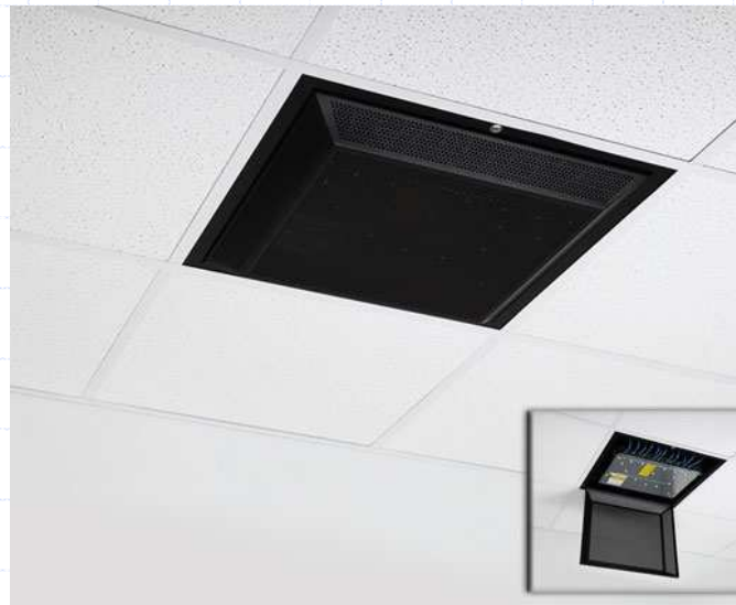
Ceiling Switch enclosure
